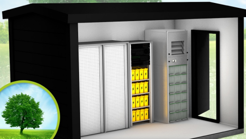
EC Air 60-L PCM Inside shelter
